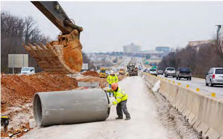
APAC-Central, Inc. crews worked through the winter months and are now approaching the end of a $10.1 million project to widen Interstate 49 to six lanes between New Hope Road and U.S. 62/102 in Rogers. The work should be complete later this year.
